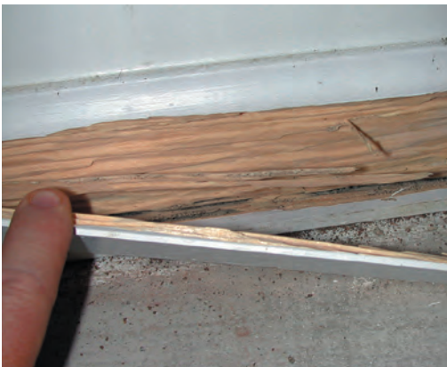
Figure 8. Subterranean termites will consume or damage structural wood (top) as well as door frames, paneling, carpet, and baseboards.
