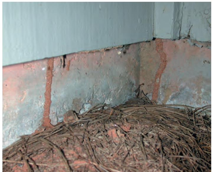
Figure 21. Property owners should keep mulch away from their building's foundation to allow inspectors to detect the presence of termites moving from the soil into the structure. In these pictures, mulch is piled next to the structure (top), and when removed exposes termites entering the structure through shelter tubes (bottom).
